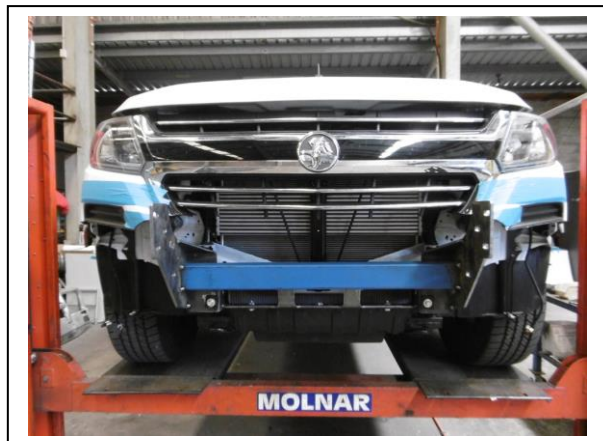
Figure 15: Cut across grille to fit over steel mount leaving grille mount on grille.
